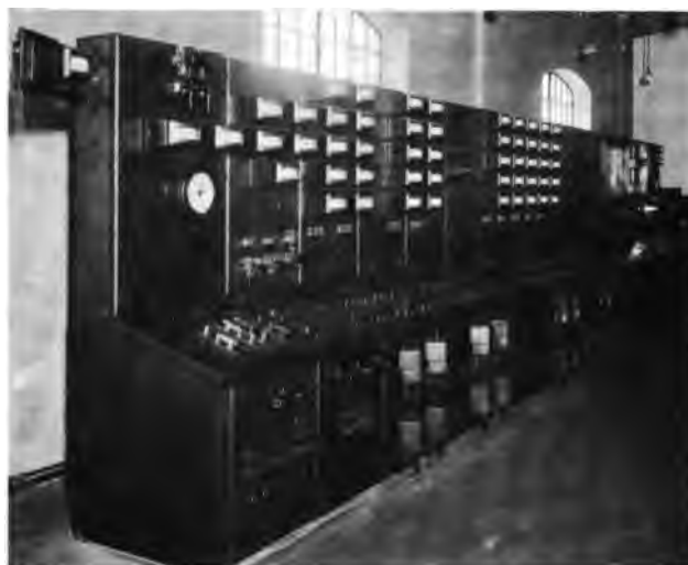
Fig. 4. Remote Control Equipment in High-Tension Station.‡
